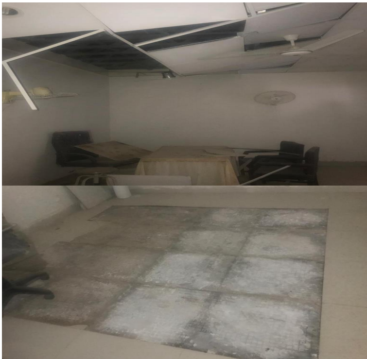
Picture-21 (Trauma center Gaularchi Dist: Badin) Roof leaked due to rain & also tile broken
