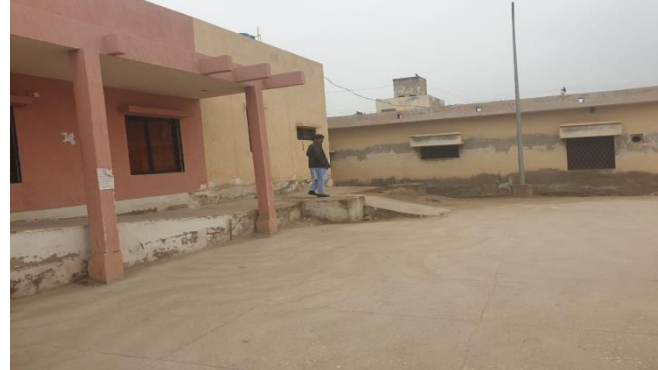
Picture-26 (Trauma center KN Shah Dist: Dadu) Improper slope and poor plinth work
