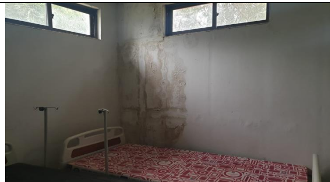
Picture-22 (Trauma center Johi Dist: Dadu) Seepage on walls and Washroom without plumbing accessories
