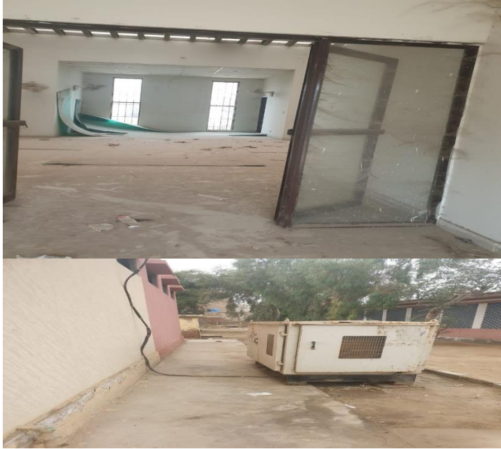
Picture-23 (Trauma center Mehar Dist: Dadu Broken shade at entrance and cracks on base
