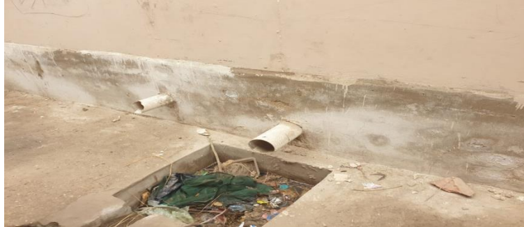
Picture-25 (Trauma center Dokri Dist: Larkana) Drainage lines not properly constructed
